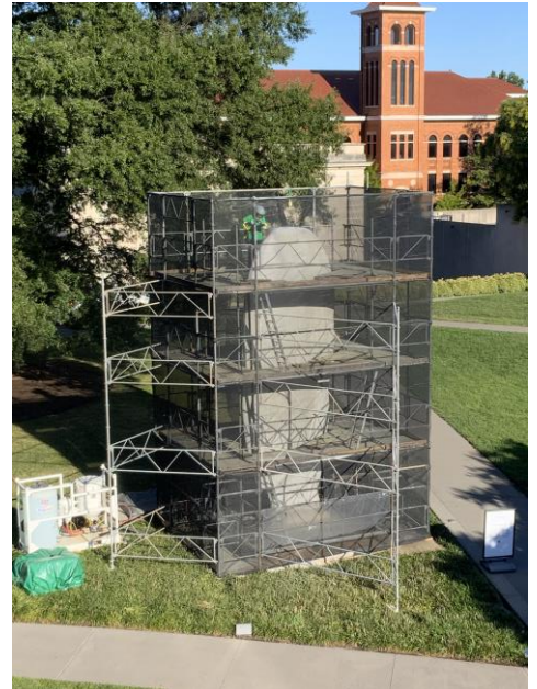
Chloe, surrounded by scaffolding that permitted access to all areas of the sculpture for treatment.
